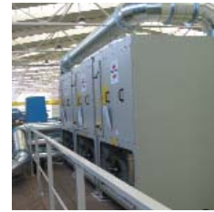
Surface filters, L-CUT
