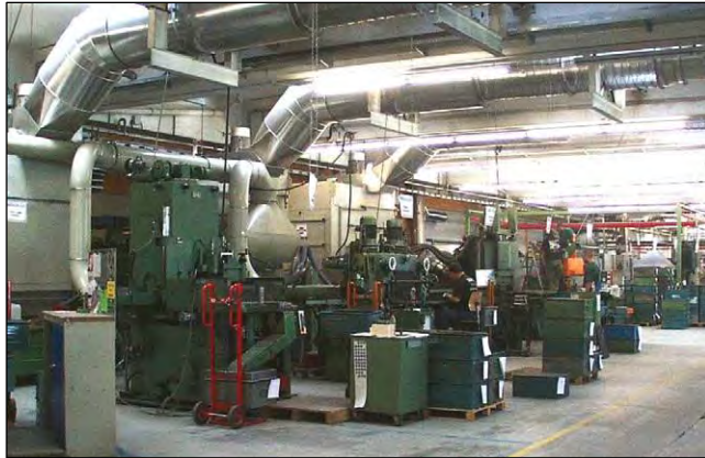
Dust Collectors are integrated in the production process
